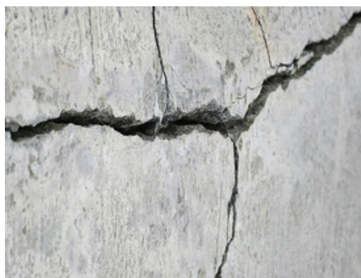
© stone crack, Fotolia #3669926
